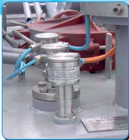
Klay Pressure transmitters on inland chemical tanker
